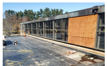
Above: New roofing at kitchen area, removed mechanical louver at existing gymnasium.
