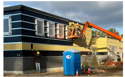
Above: Installing insulation at the hardy panel siding locations at Band corner of building.
